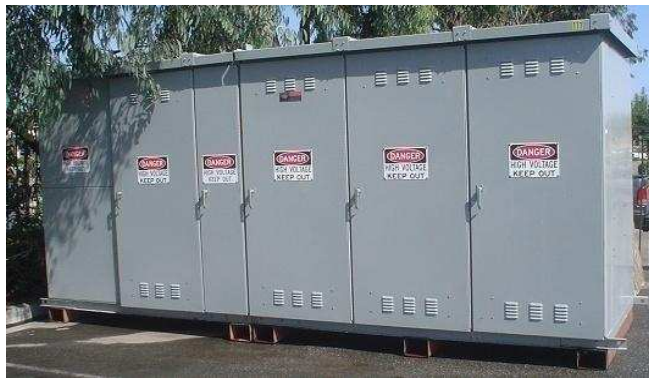
UNIT #117 w/ #116 Attached as MAIN making a 4 gang line
